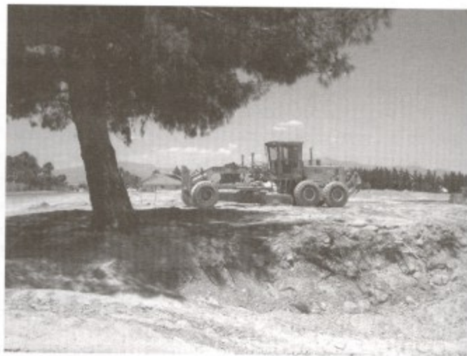
Root system damage during construction. Note rooting depth.
